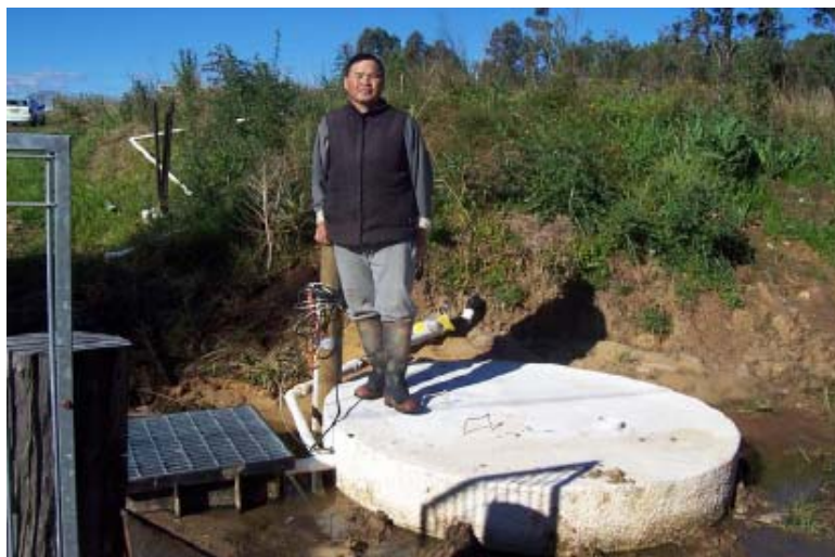
Figure 4: The IWRS system installation.
